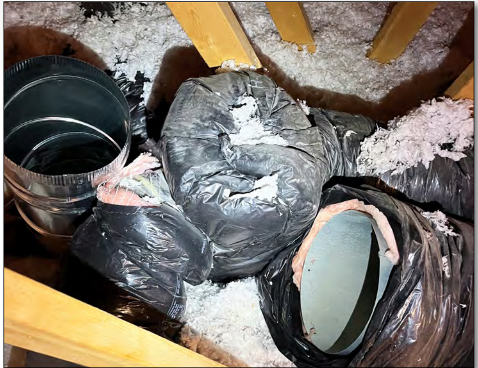
A supply duct in an attic was taken apart to remove a pinch point in the flexible duct. Then the supply duct was sealed properly.
