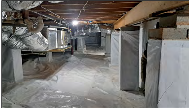
Crawlspace encapsulation is just one of the many services Progressive has to help customers decide what to buy and when.
